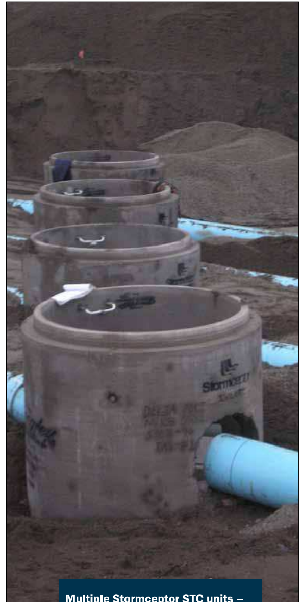
Multiple Stormceptor STC units – provides stormwater treatment and spill capture at the Delta Port in Vancouver, British Columbia, Canada
