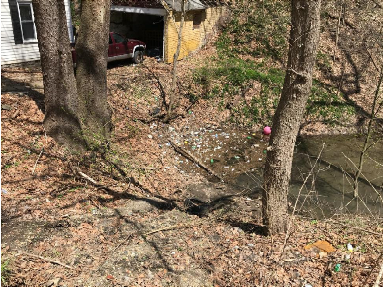
Outfall #7 of UNT #7 to the Monongahela River along Tyrol Boulevard 24" RCP (submerged in water/sediment at toe of slope)
