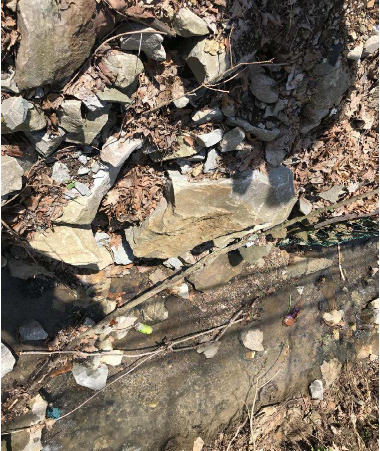
Outfall #6 of UNT #2 to the Monongahela River along Tyrol Boulevard 18" RCP (covered with riprap)
