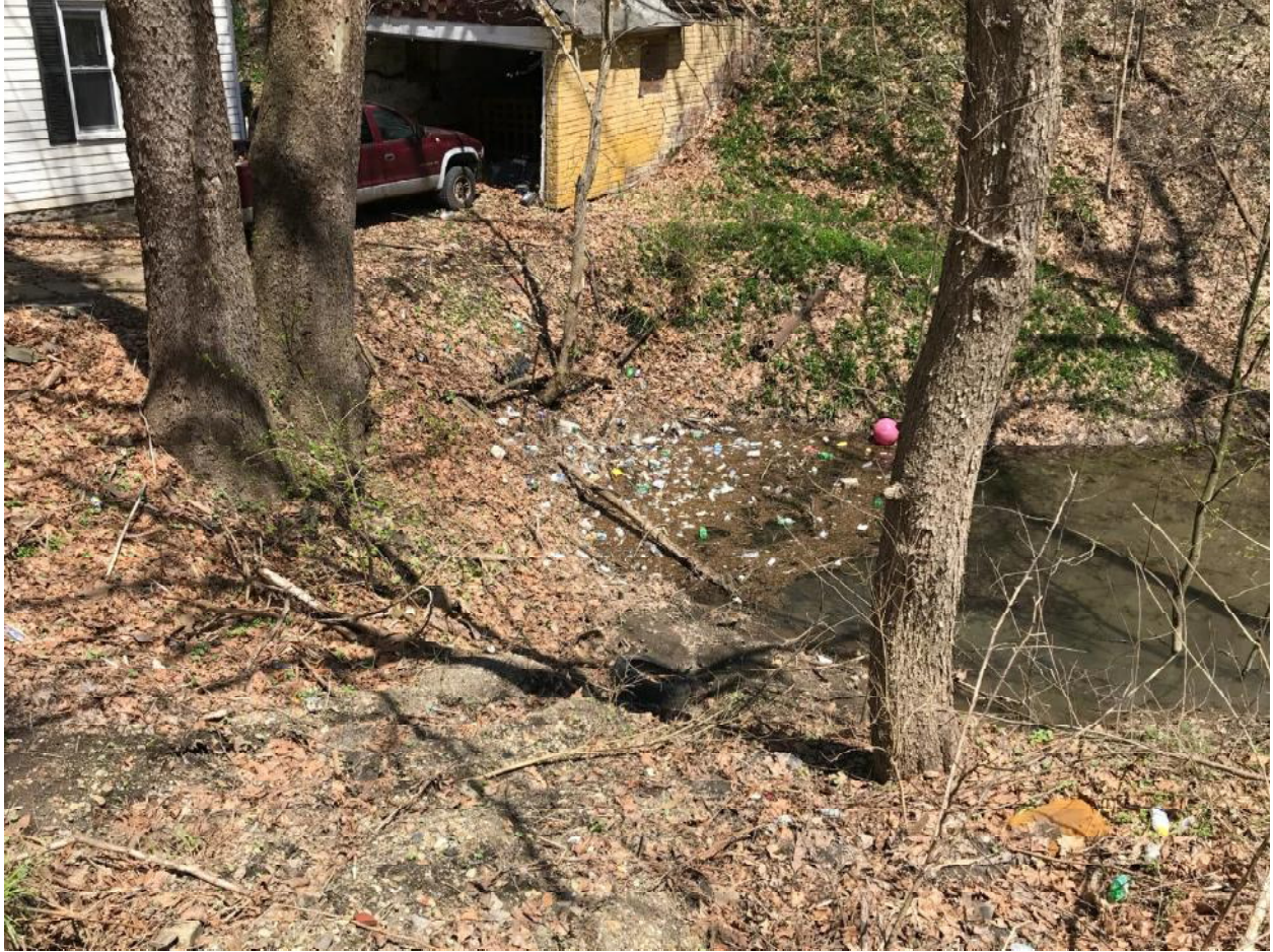
Outfall #7 of UNT #7 to the Monongahela River along Tyrol Boulevard 24" RCP (submerged in water/sediment at toe of slope)
