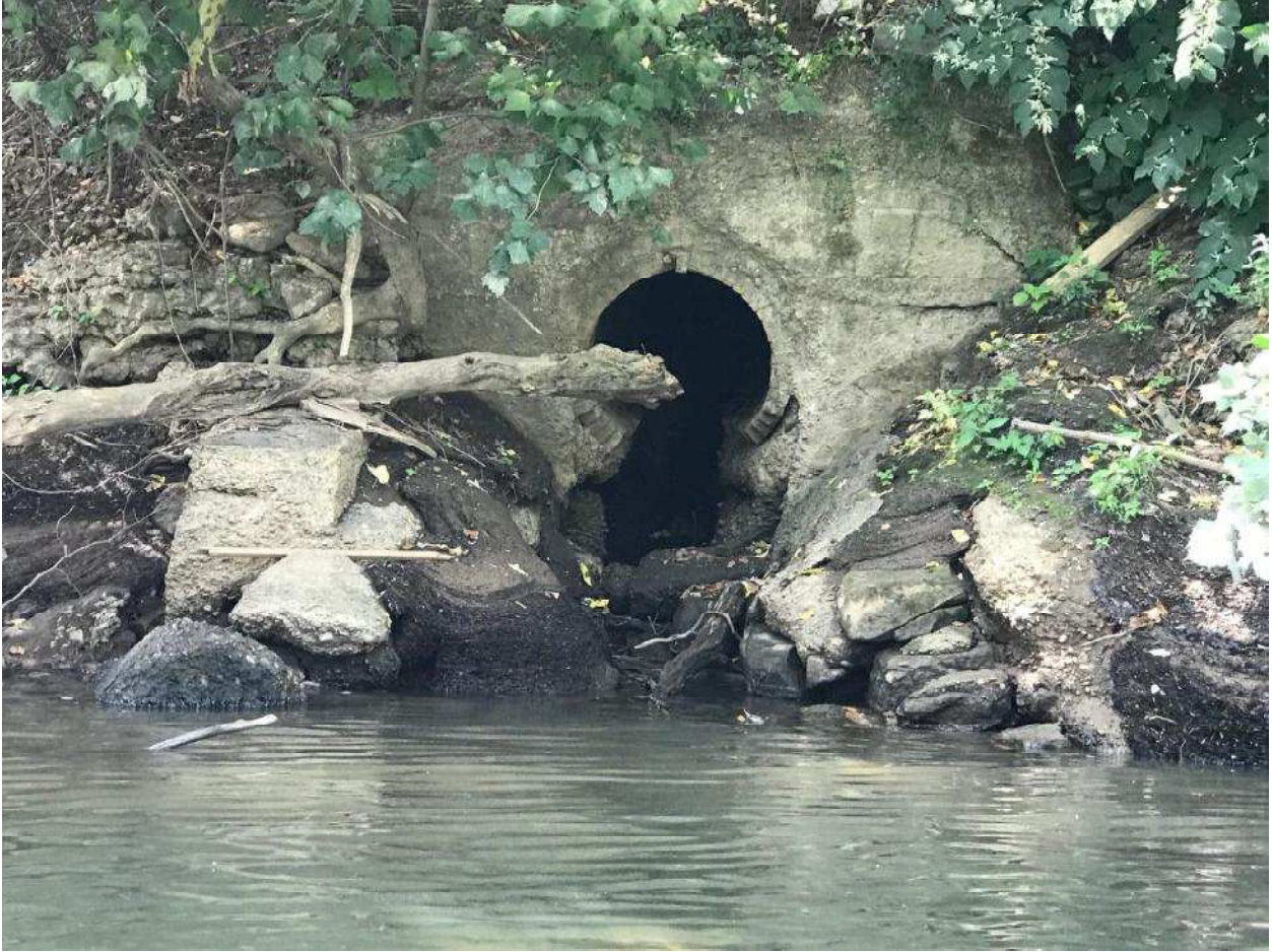
New Outfall E of the Monongahela River. Note invert of pipe eroded away.
