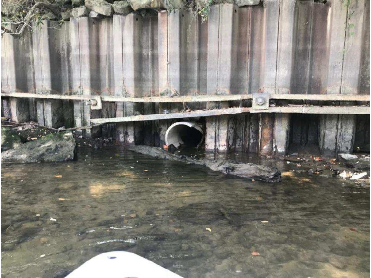
Outfall #CS102 of the Monongahela River.
