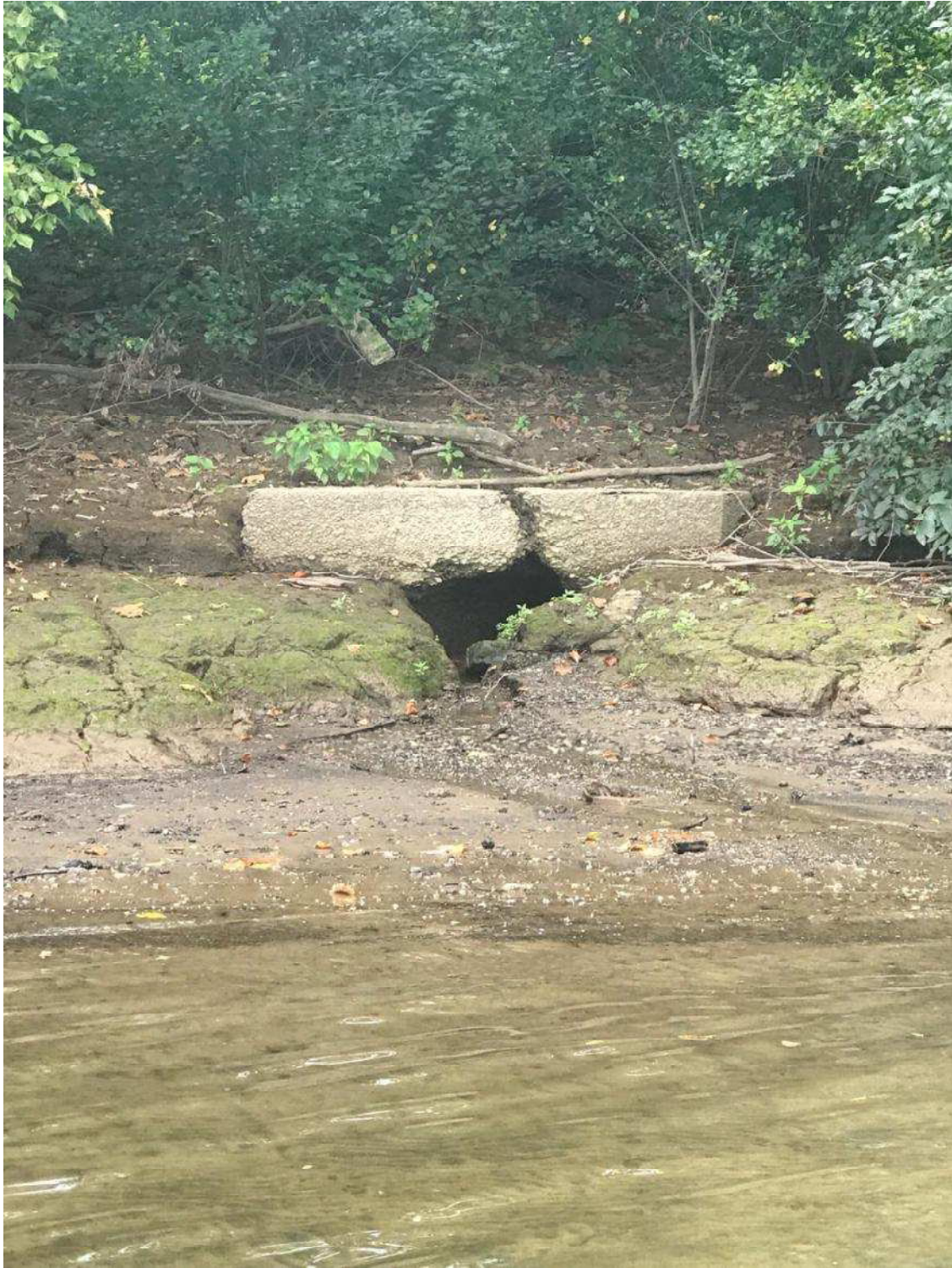
Outfall #CS006 of the Monongahela River. Note large area of sediment deposition from the river.
