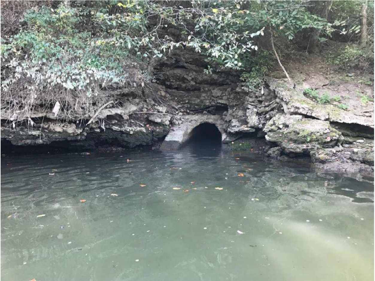
Outfall #CS003 of the Monongahela River
