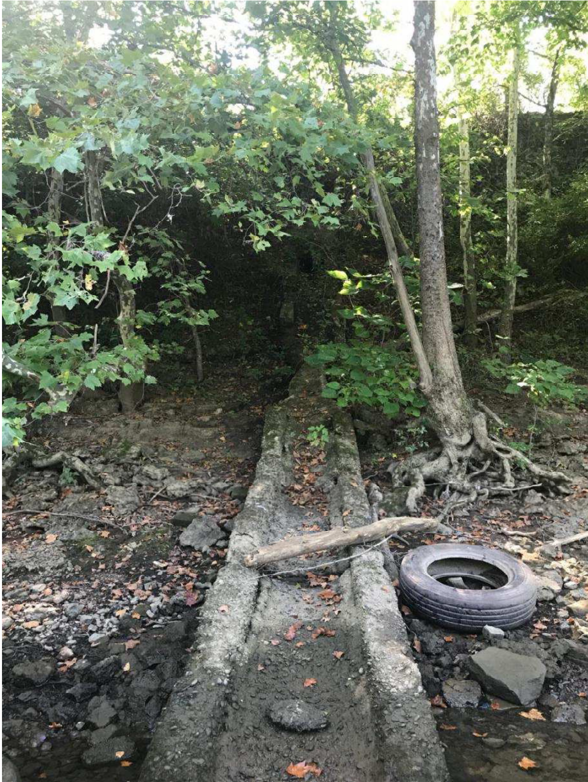
New Outfall B of the Monongahela River. Note existing concrete outlet channel
