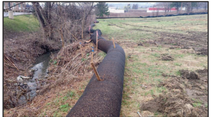
Figure 7: Filter sock used to provide erosion and sediment control (Source: Westmoreland Conservation District)
