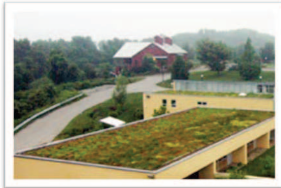
The 1st green roof (above) in Westmoreland County is located at the County Conservation District's office. This installation was part of extensive sustainable stormwater retrofit solutions across the site. Photo: wcdpa.com
