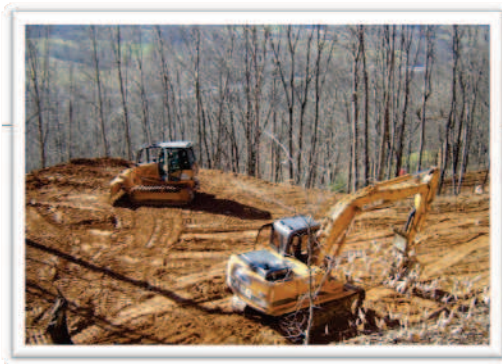
Areas that are disturbed during grading (above) are prone to soil erosion and compaction.
