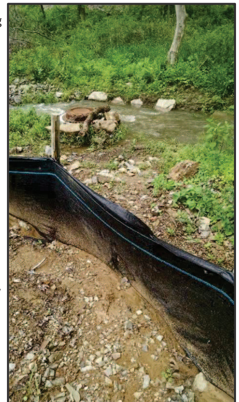
Figure 8: A damaged silt fence which is supposed to provide erosion and sediment control where soil is being disturbed by construction (Source: Allegheny County Conservation District)
